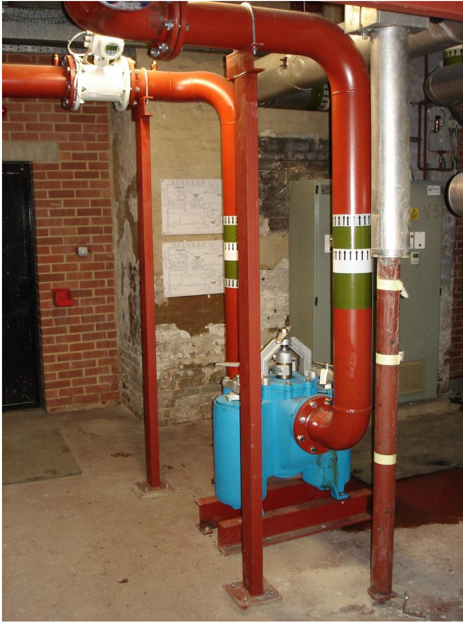
New duplex strainer and (top left) electronic flow meter serving Poultry Market. The flow meter is linked to the City's Building Management System, allowing the flow rate to be monitored and recorded continuously. There are separate meters for East and West Markets.
