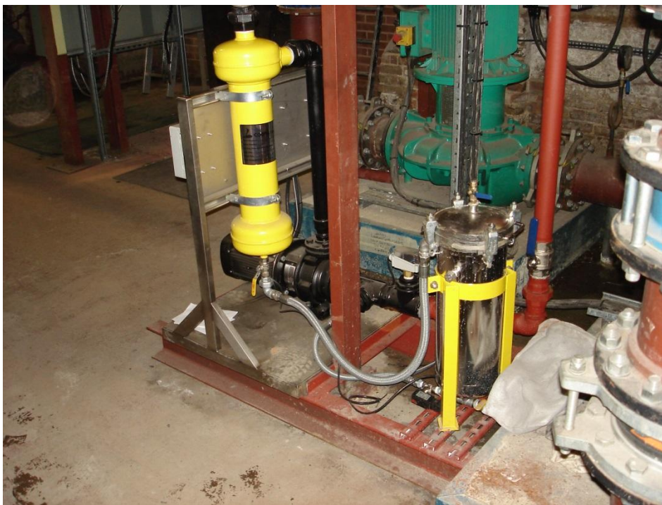
New sidestream filtration unit. This is a cyclone type cleaner; dirt collects in a bag within the container on the right and requires periodic emptying. The green pump seen at the rear is one of the two main cooling tower pumps.
